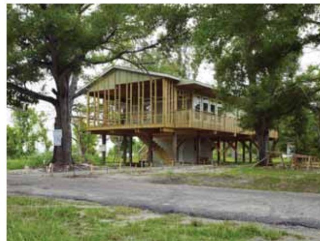
FIGURE 46. New houses in the neighborhood, constructed to meet revised base flood elevations at a range of heights. Image credits: from top left to bottom right: Top, GCCDS, Jonah Reeves, Leslie Schwarz. Middle, Leslie Schwarz, Jonah Reeves, Leslie Schwarz. Bottom, Alan Karchmer.
