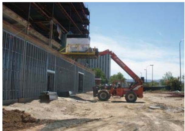
(Figs. 6-8) Component pods are delivered by truck and lifted into the structure.
