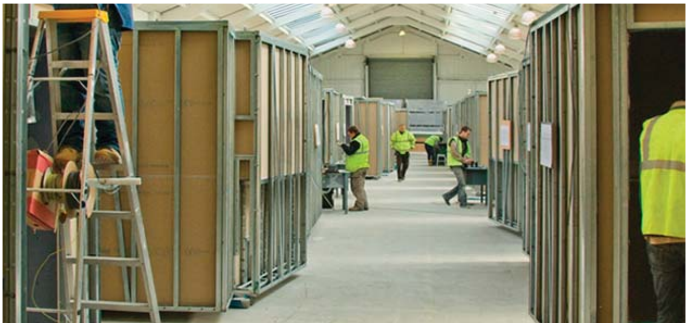
(Fig.9) Pods can be easily wired and plumbed due to greater access and a factory setting which encourages quality and efficiency.
