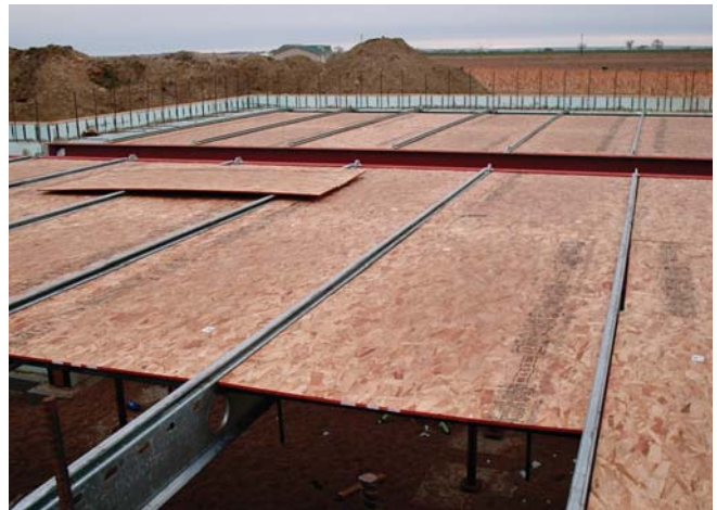
(Fig.7) The steel joists are spaced 49" on center to allow for 4x8 sheets of plywood to slide in between. The plywood is removed after the concrete is cured.
