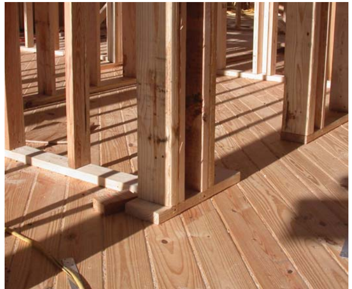
(FIG.A) TONGUE AND GROOVE FLOORING This 2x6 southern yellow pine floor will be sanded and finished with a stain or sealer.
