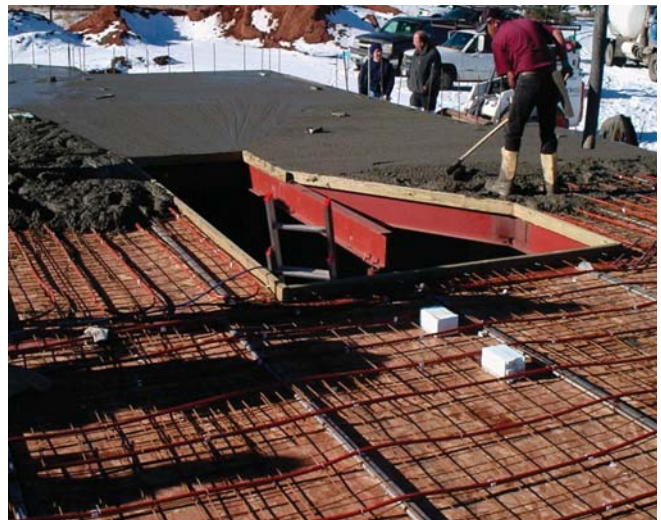
(Fig.8) A professional concrete installer spreads concrete over the formwork. Here, rebar is used instead of steel mesh for reinforcement.
