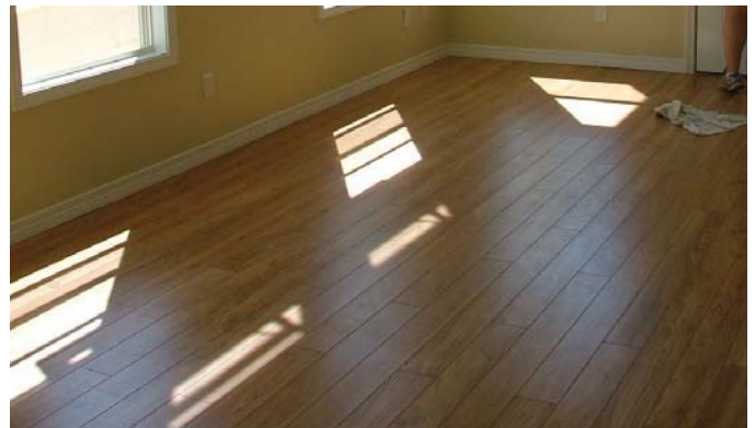
(FIG.B) FINISH MATERIALS are applied on top of the subfloor. In the past decade more sustainable finish materials have become widely available.
