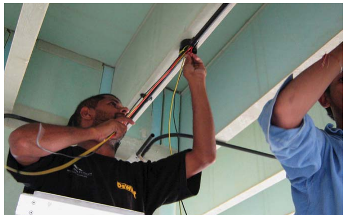
(FIG.C) INSTALLING electrical, mechanical, plumbing, or other systems may require planning ahead. Coordinate with tradespeople to avoid delays or cost overruns.
