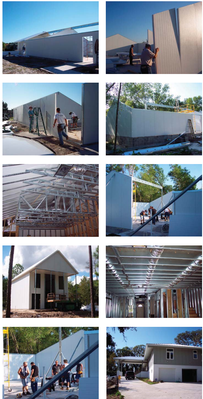
(Fig.19) Construction photos from several homes built using steel SIPs by Marquis Construction & Development.
