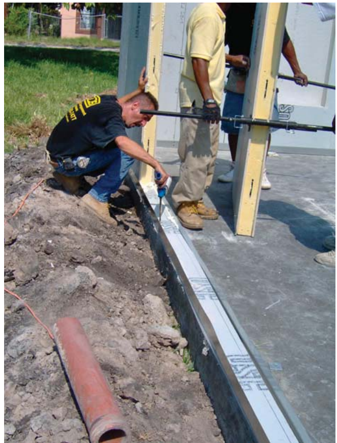
(Fig.14) A worker installs fiber cement panels in a house in Orlando, FL.
