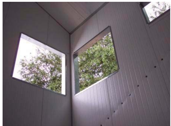
(Fig.16) Metal SIP corner showing window openings cased out using galvanized steel channels.
