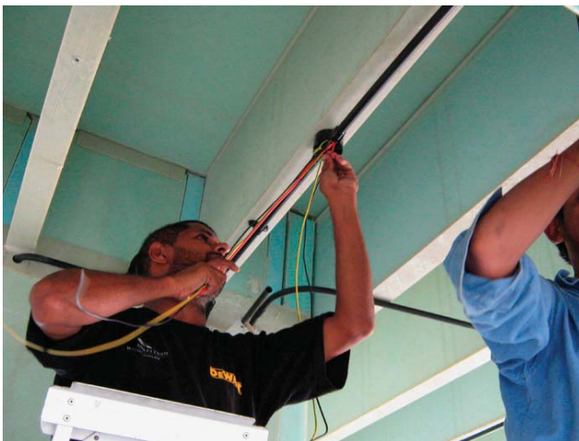
(Fig.15) A worker installs wiring in a house built using InnoVida fiber-reinforced plastic panels in Dubai, UAE.
