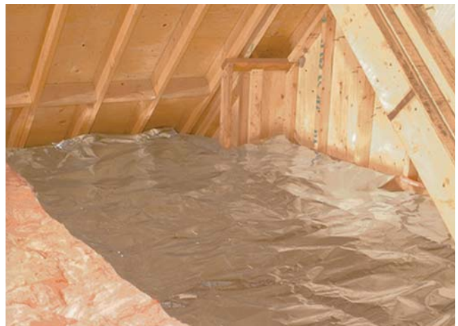
(Fig. 3) Rolled-out foil covers the attic floor insulation. Little fastening is needed to keep the product in place. Note the reflective side faces the interior.
