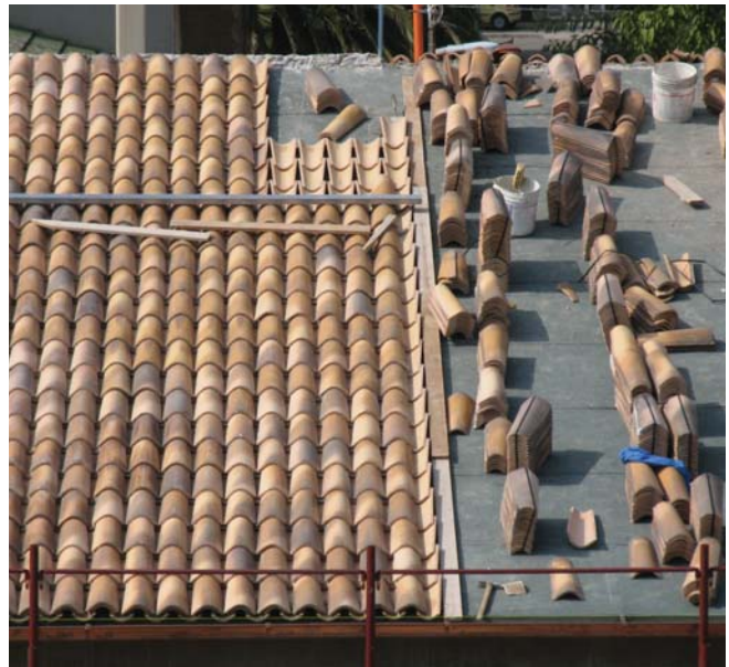
(Fig.17) Tile roofs require a thicker roof deck to support the added weight of the tiles. These tiles are being installed using mortar to hold them in place.
