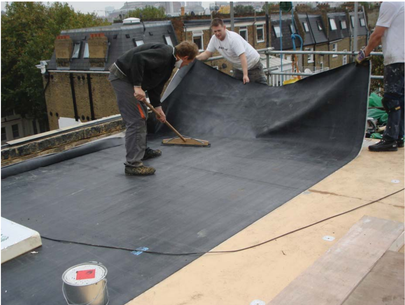
(Fig.21) Installing an EPDM roofing membrane is a relatively straightforward task, but requires care and the appropriate adhesives.
