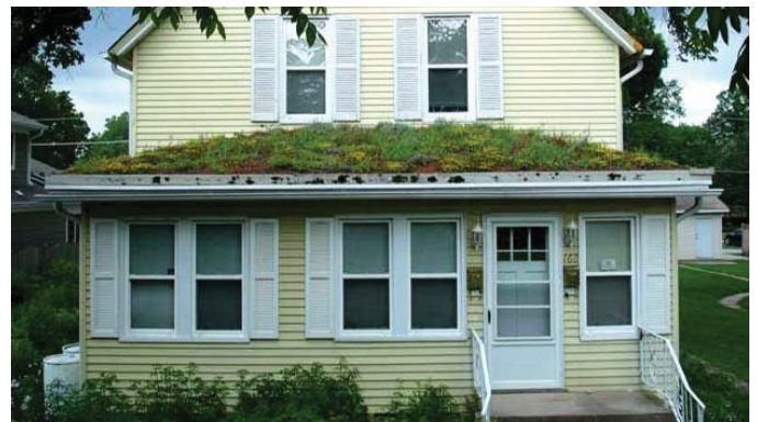
(FIG.C) Green Roofs are an unusual option in residential construction. The larger the area, the greater the insulative impact.
