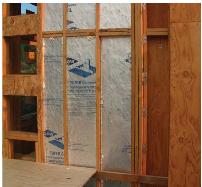
(Fig. 7) Radiant barriers are commonly used in the attic, but can be installed in other locations. This image shows radiant barrier backed plywood being used inside a wall cavity.
