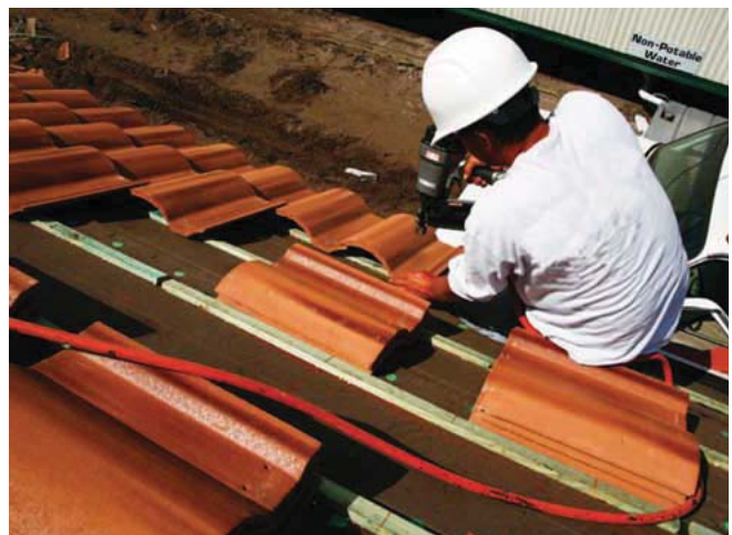
(Fig.18) A preferred method for securing tiles in a high wind zone is to nail them to sleepers. This is a stronger connection that is less likely to fail over time and helps prevent uplift.
