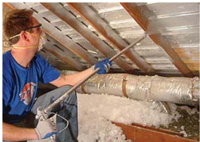
(Fig. 4) A spray-coated radiant barrier can be applied to the underside of the roof decking.
