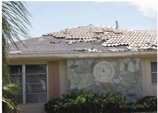
(Fig.19) Tiles ripped from a roof in a storm can become projectiles likely to damage other area of the roof. They can also cause damage to persons and structures.
