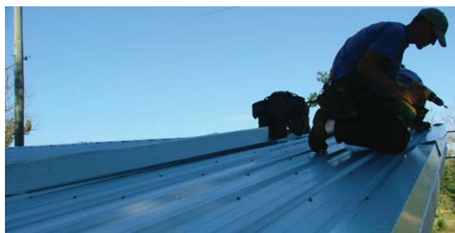
(Fig.11) After the sheet metal is in place, contractors install the top rake cap.
