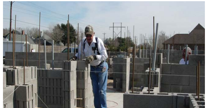
(FIG.B) CONCRETE MASONRY UNITS (CMU) are easy to stack by hand. Vertical reinforcement is set into the foundation and continues through the wall.
