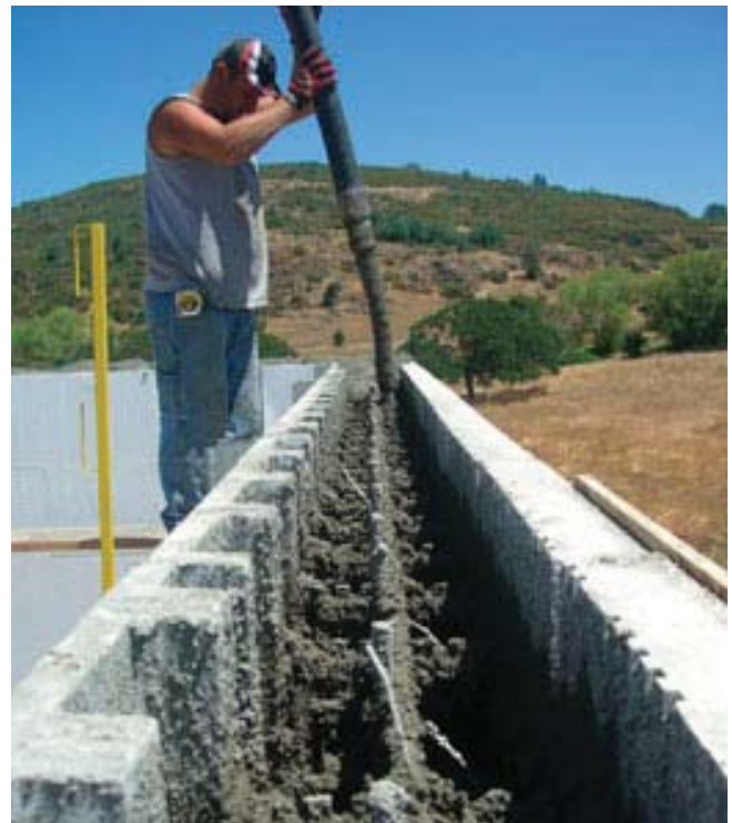
(Fig. 7) ICF walls are poured with concrete in 4' lifts, horizontally, with a concrete pump.
