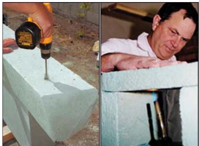
(Fig. 18) Vertical holes are drilled through the blocks for reinforcing bars. After the bars are set, the holes are filled with structural mortar.
