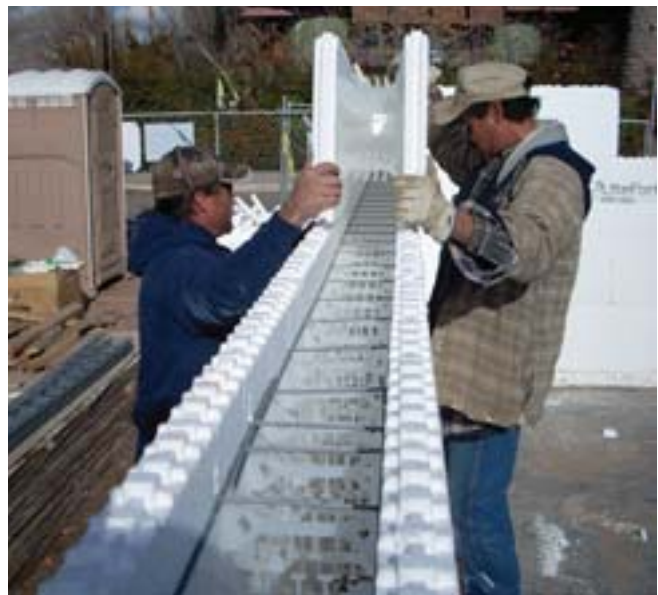
(Fig. 4) A small crew of just a few laborers is needed to stack the formwork.
